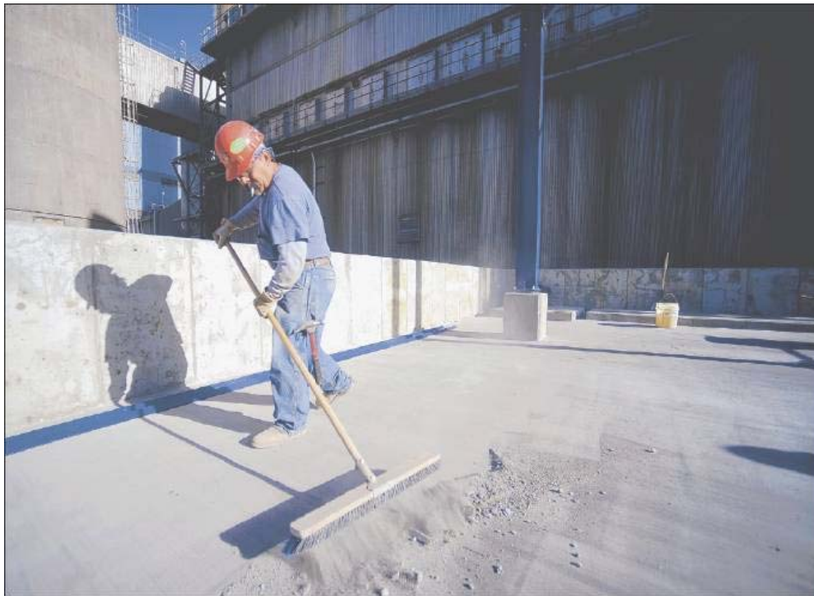
Darrol Vigil of Industrial Construction Managers Inc. in Pueblo swept an area of the Martin Drake Power Plant on Monday that will eventually become a solvent process system.
